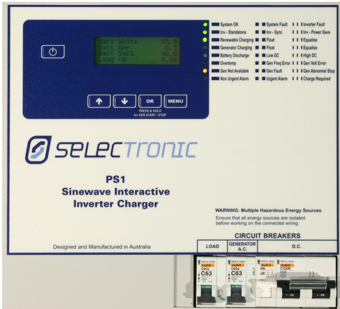
Figure 5 PS1 Circuit Breakers
